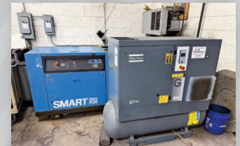
Air Compressor System
