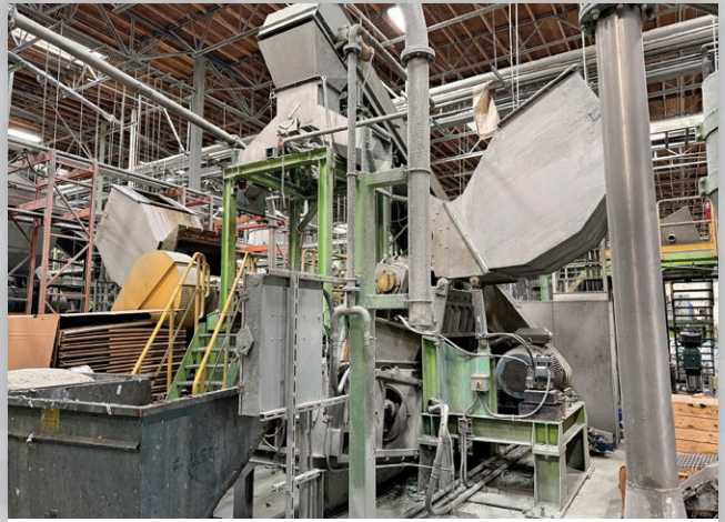
(2) 150-KW (Approx.) Sorema Previero MU-812H Wet Grinders w/ Centrifugal Drying Systems
