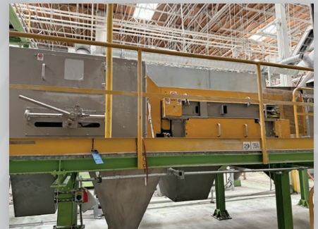
Sorema 4,500 Kg/Hr Eddy Current System on clear line
