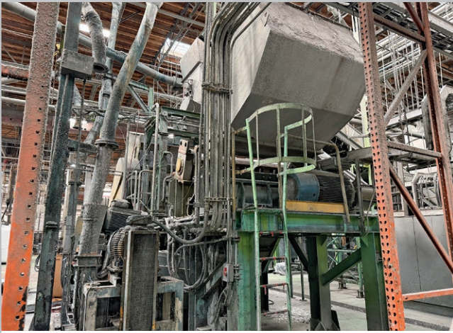
(2) 250-KW (Approx.) Sorema Previero MU-920PRH Wet Grinders w/ Centrifugal Drying Systems
