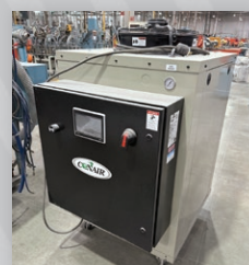
(5) Thermal Care Chillers
